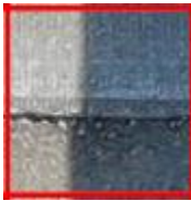
Figure 4. Example of road to gravel transition (counted as crack)
